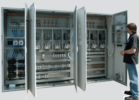
Control panel manufactured by Colt undergoing final inspection
